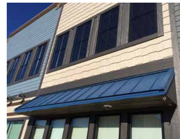
This property uses Diamond Kote Terra Bronze RigidStack siding, sand board, and batten with white nail fin trim and nail fin outside corners. At left, this storefront uses Oyster Shell Staggered RigidShakes, Smoky Ash RigidStack siding, and nail fin trim prefinished in coffee.
